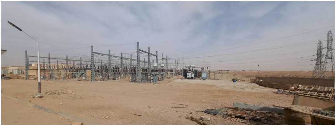
Figure II.4 : photo de l'étage 60/30Kv post GHARDAIA.
