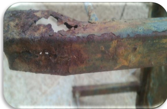
Figure N°13: Fissure de CSC [31].
