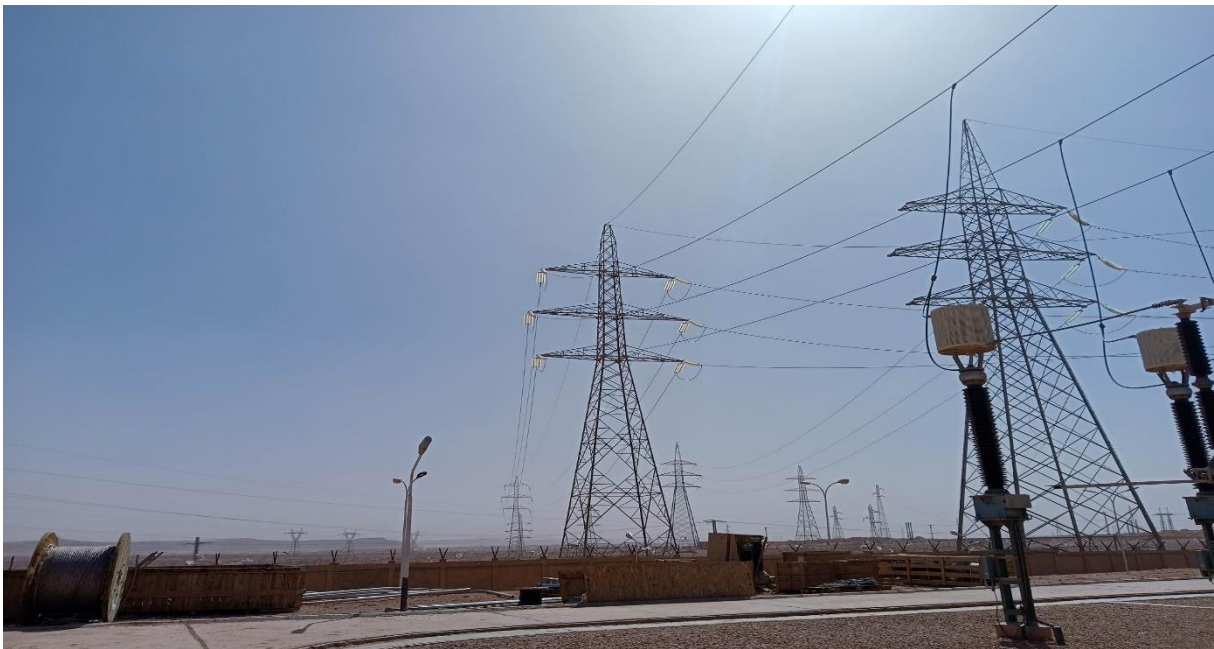
Figure II.4 : Ligne haute tension.
