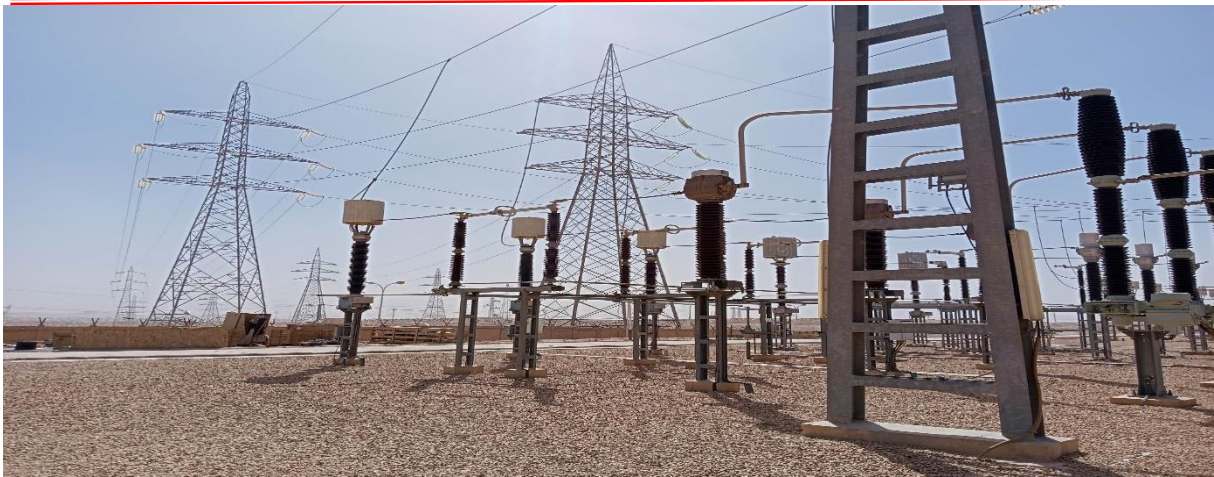
Figure II.4 : Ligne haute tension.
