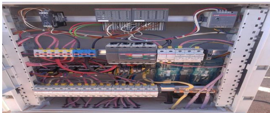
Figure III.10 : photo interne de boit de raccordement
