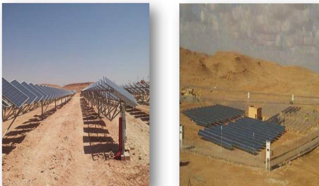
Figure III.2 : Installation photovoltaïque d'OUED NECHOU Ghardaïa.
