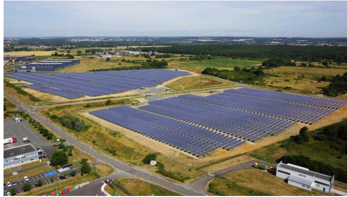
Fig III.1 le Champ de Photovoltaïque [13]
