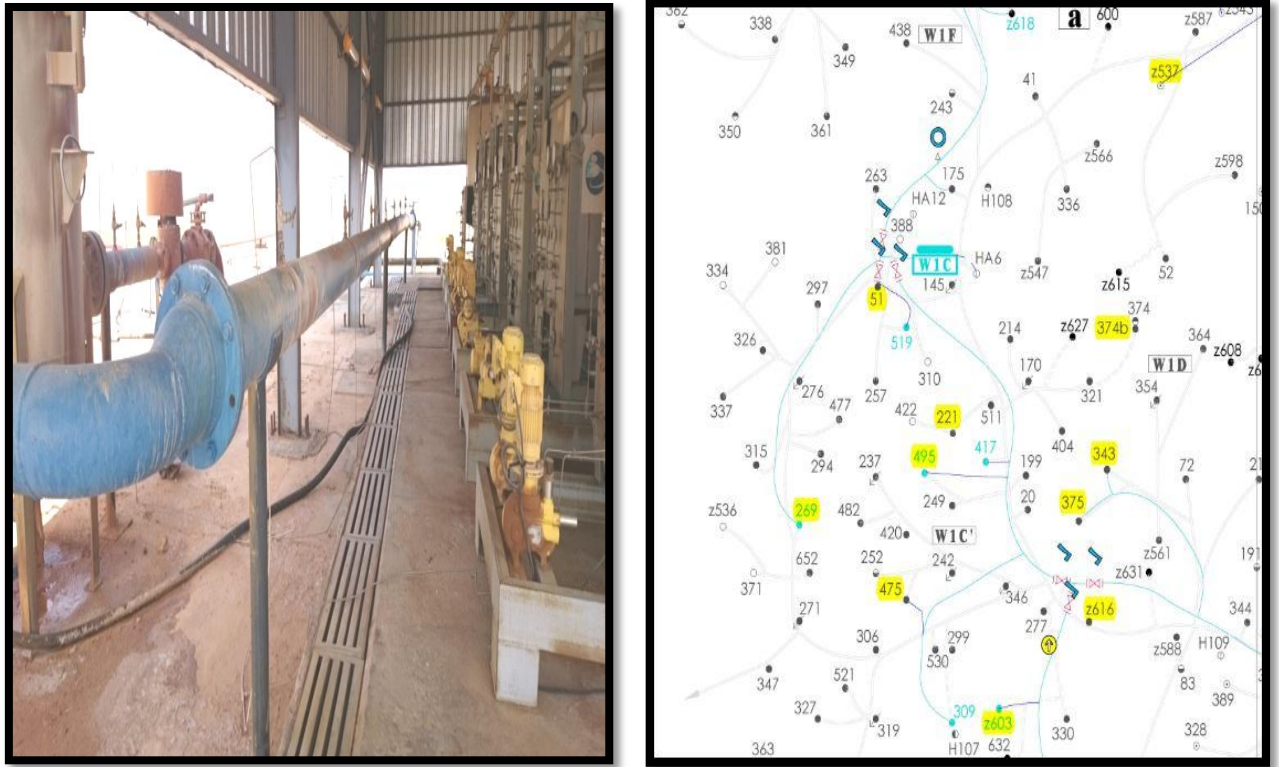
Figure N° VI.6: Station de traitement WIC.
