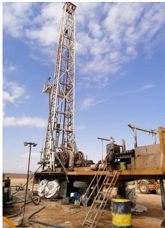
Figure II.4 : Le mât de forage.
