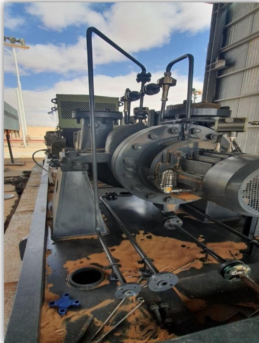
Figure III.12 Pompe haute pression
