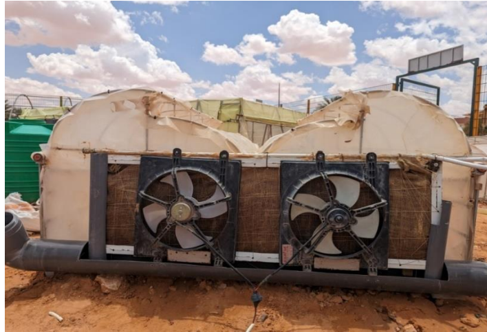
Figure III-23: the external view of an experimental fan-pad cooling system.
