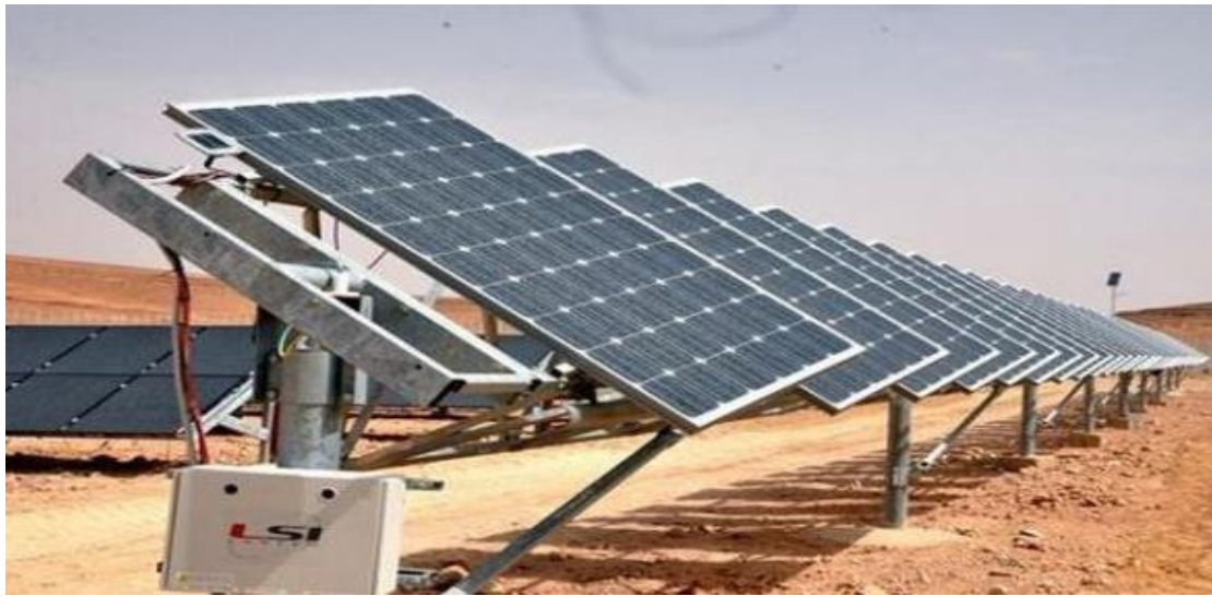
Figure I. 9. Station photovoltaïque d'Oued Nechou
