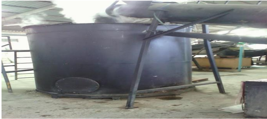
Figure I.6: Cuve de lavage [11].
