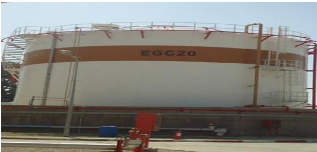
Figure 49 : Bac de stockage fuel EGC20 [7]
